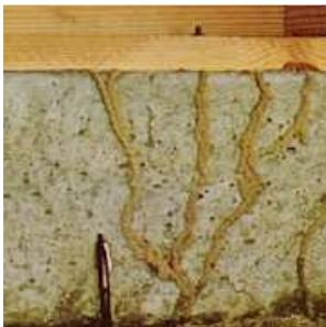
Subterranean Termite Mud Tubes
