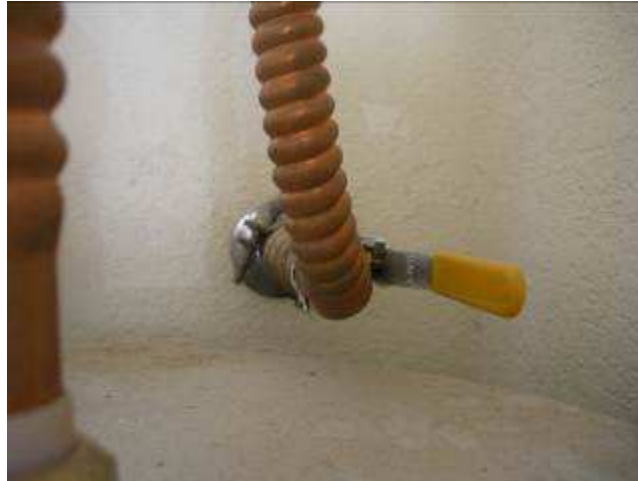
Photo 6: Cold Water Inlet Pipe and Ball Valve Shut-off)
