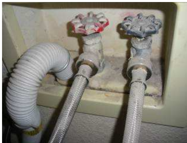
Photo 5: Cold and Hot Water Supply Valves
